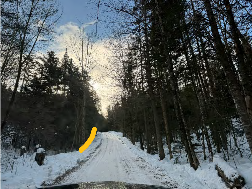
16735 before 1 - stone line ditch with erosion stone left side to top of hill
